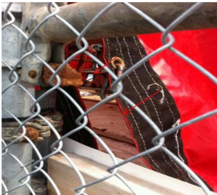
Fig. 3: A close-up view of a large gap in a “containment structure” where power tools are being used to remove lead-bearing materials during the MCRRP.
