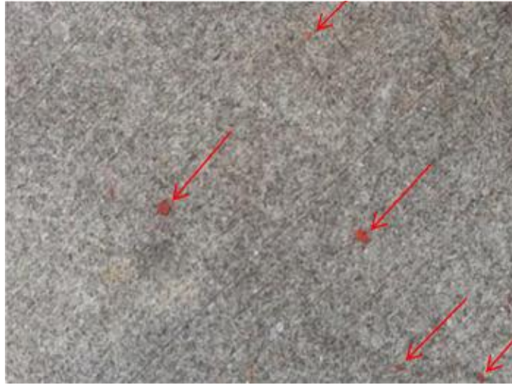
Fig. 4: Photograph of lead-bearing paint chips on the public sidewalk on the east side of the Bridge under lead containment structure.
