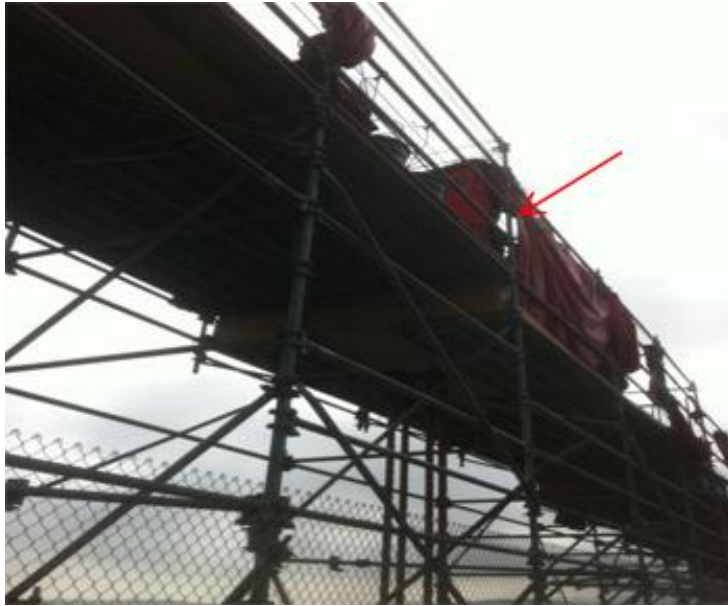
Fig. 1: Picture taken of “containment structure” at east side of Bridge. At the arrow you can see the sky through the structure where a roof should be blocking this view. Curtains are not fastened together resulting in large gaps.
